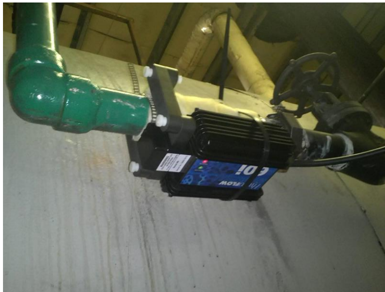
HydroFLOW 60i on pipe feeding the steam boiler
