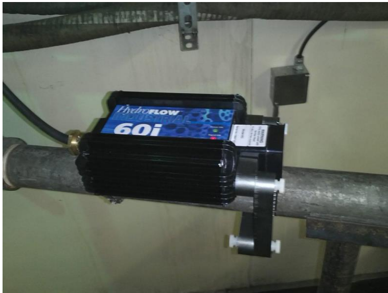
HydroFLOW 60i on water line from softener
